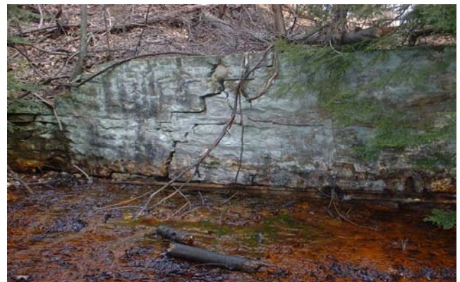
Opening of the General Refractory Mine located in Bradford Township. Only the top of the opening is visible due to iron precipitate.
